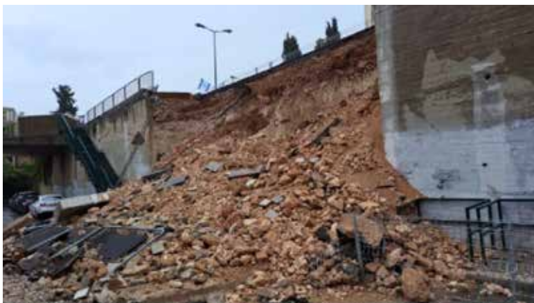
Walls as a nuisance: collapse of a retaining wall on Yad Levanim Street in Haifa in 2023; its restoration is still in progress
